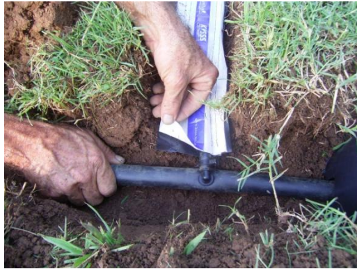
Photo 1: KISS Flat must be installed with the black base layer of plastic down and the white geo-textile facing up.
