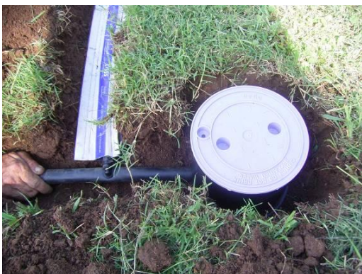
Cover flush valve with cap and back fill soil (cap remains visible at ground level)
